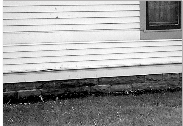
A replacement foundation should be similar to an original foundation such as this one.
