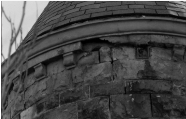
A porous sandstone cornice is prone to deterioration, which has accelerated mortar failure.
