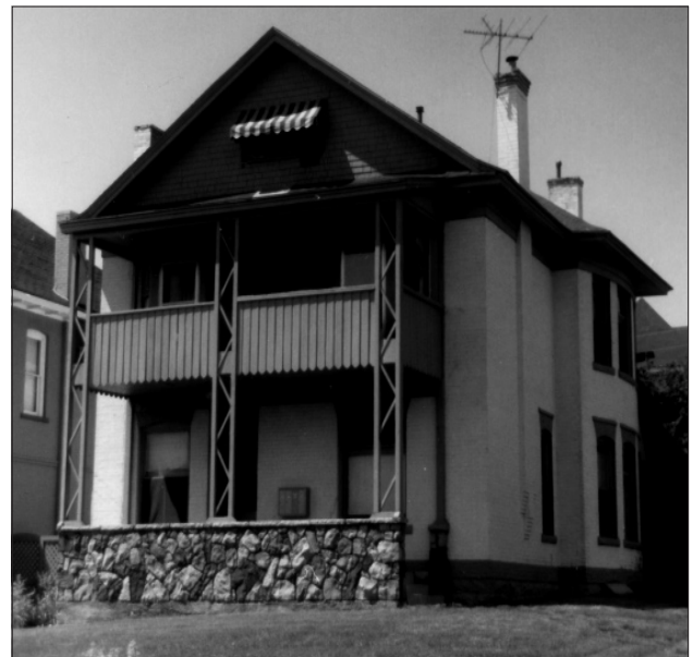
This porch has been altered. As a result, its historic character is compromised.
