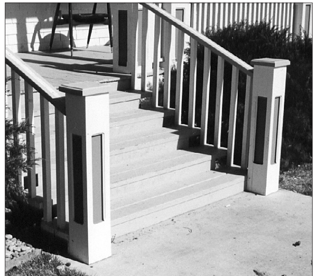
It is preferred to repair any deteriorated portions of a porch, rather than replacing the porch altogether.
