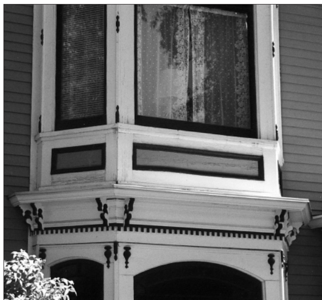
The ornamentation within this original two-story bay window helps retain the integrity of the house.
