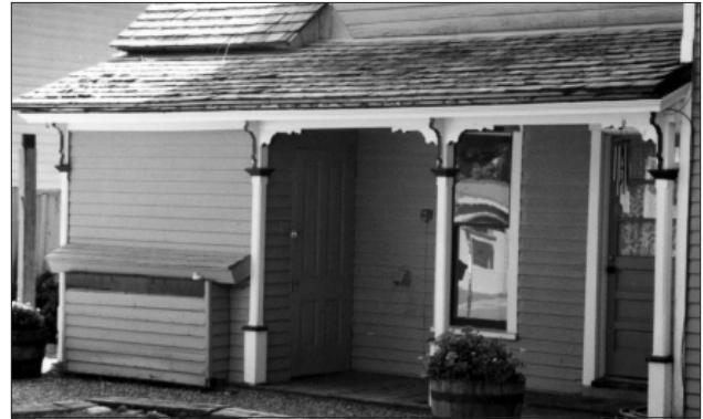
This reroofing job maintains the historic character of the house by using traditional wooden shingles. Note the proper technique of attaching shingles to battens for proper ventilation to enable moisture evaporation, prolonging the life of the roof.
