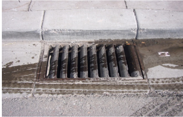
Figure 4.6 Grate Inlet used in City of Aspen
