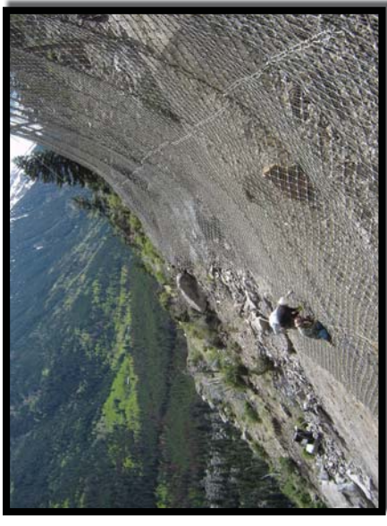
Rockfall Mesh on a Slope
